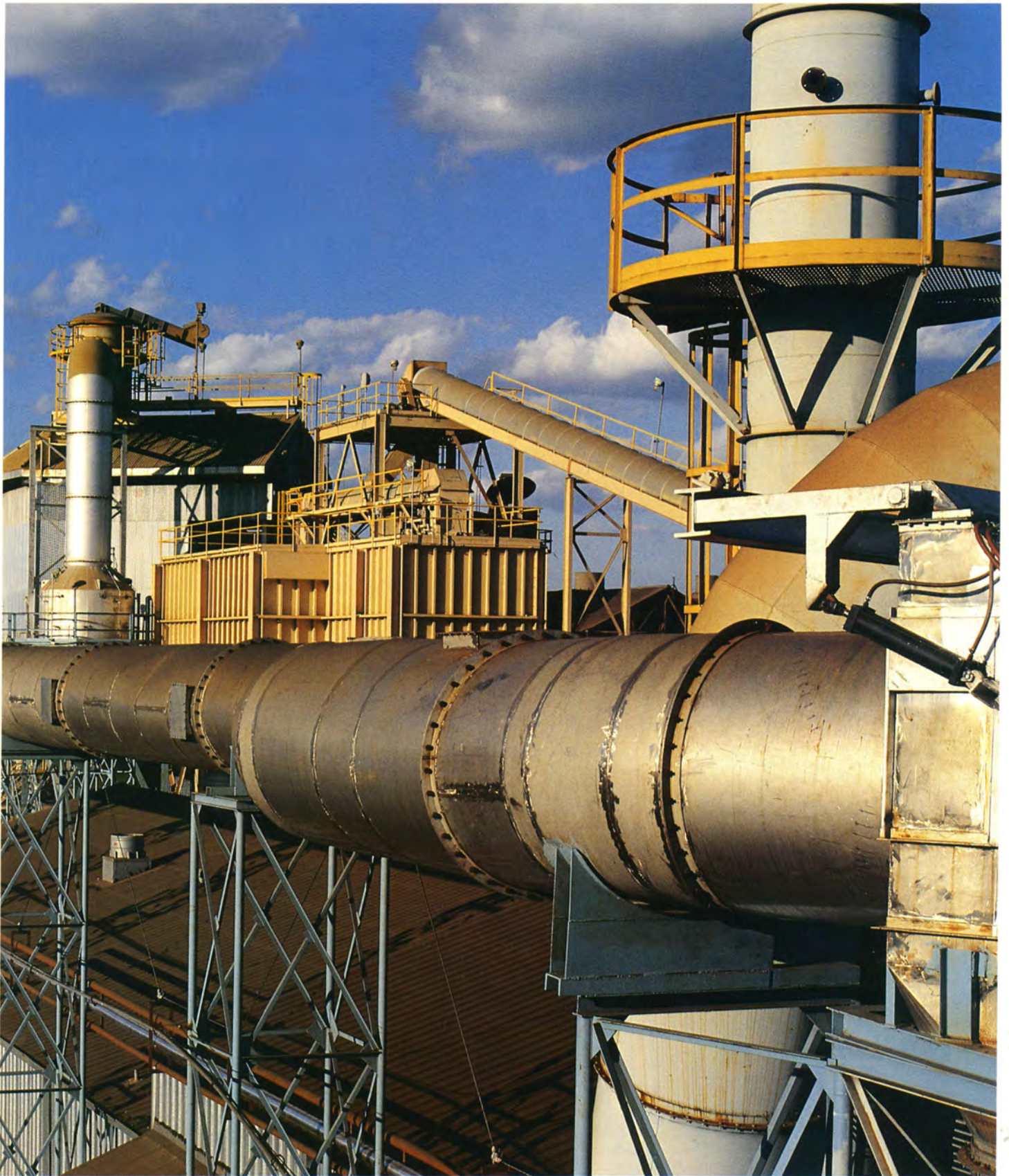
A $3.2 million melting system was installed in the foundry operations in 1981, increasing the main bay foundry's melting capacity from 25 to 35 tons per hour, and with the added capability of melting 50 tons of iron per hour in the future. It exceeds state and federal air quality codes.
