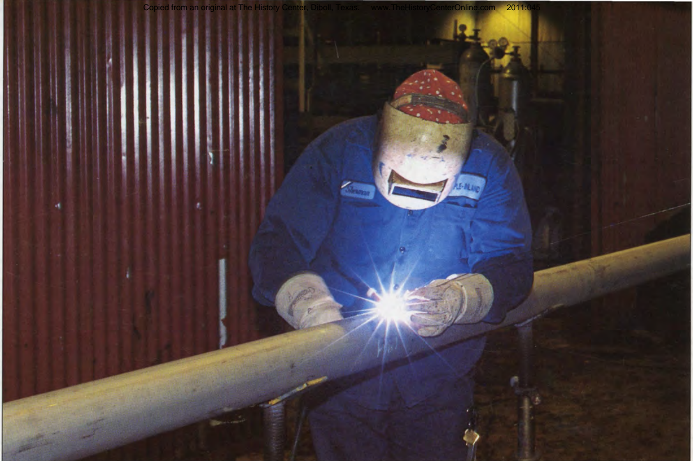
Sherman Allen, specialist welder at Temple-Inland's Fiber Products Operation, is shown welding a 4-inch stainless steel water line during the plant's scheduled shutdown in October.
