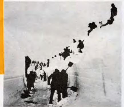
Below —Shovellers cleaning up an open cut after the machines have driven through. Notice the snow depth.
