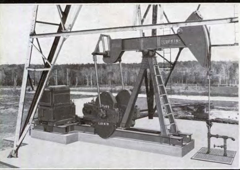
Stanolind Oil & Gas Co., Siler Lease, White and Walker Surveys in Carlisle District, East Texas installation — LUFKIN Unit Assembly T.C. No. 4-11 with McCormick-Deering multi-cylinder gas engine drive.
