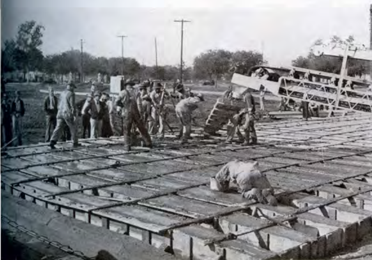
Workmen pouring concrete into forms for the 30-foot reinforced concrete piles being driven into the ground for the foundation of the $1,000,000 Texas Hall of State. —All photos by courtesy Texas Centennial Exposition.
