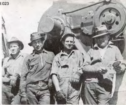
Installing Lufkin No. 41 Unit on Jergins Trust's Wright-Bloemer Lease, Mountain View Field. Buckelew, Crawford, Al Simonds, Fritz Utzerath, Asst. Supt.
