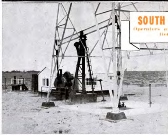
Lufkins Never Wear Out. This is a typical installation of about 40 such units transferred to Duval County by a major oil company. This unit is pumping 3 wells by means of back-crank equipment.
