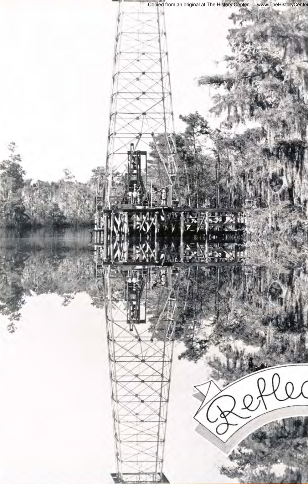
Lufkin Long Stroke Unit installation on well of a major oil operator at Westlake, La.
