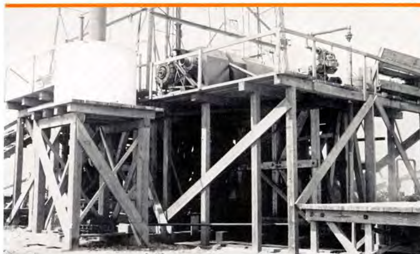
A major oil company uses a special bolted wood construction for a derrick foundation in Freeport, Texas, where a good derrick floor elevation was important because of danger from floods.
