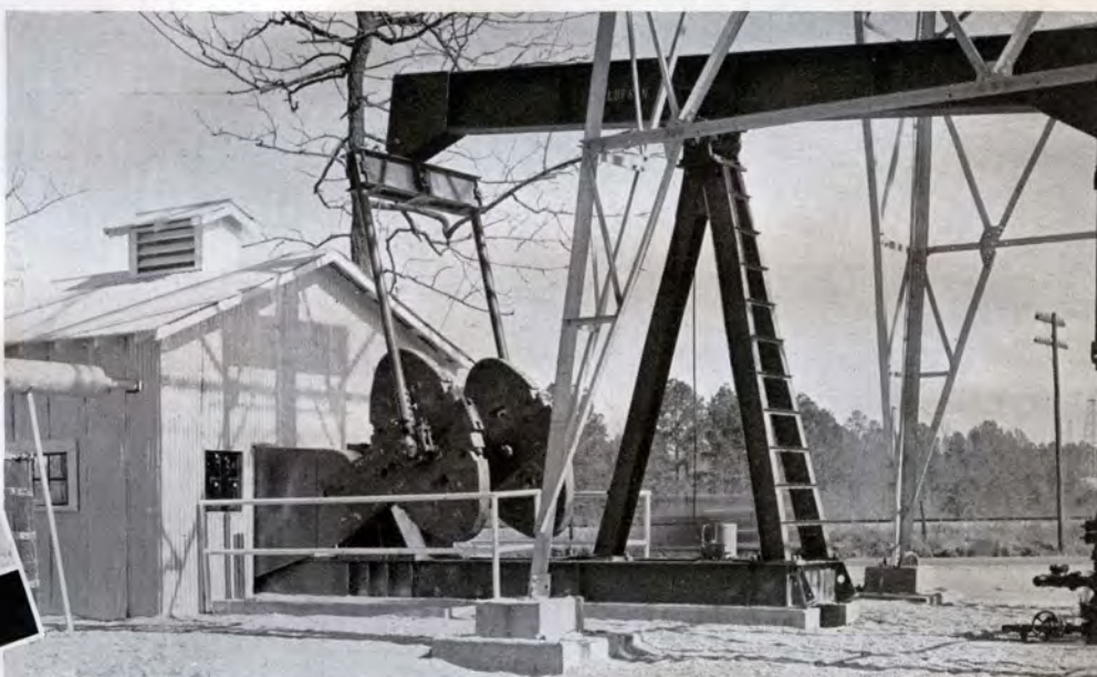
Rodessa field installation of Lufkin T.C.-54 Unit. Standard Oil Company of Louisiana.
