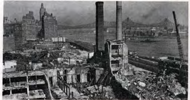
EXCAVATION of the 17-acre site began September 15, 1948, and was completed within six months. Total cost of the project will approximate $65,000,000.
