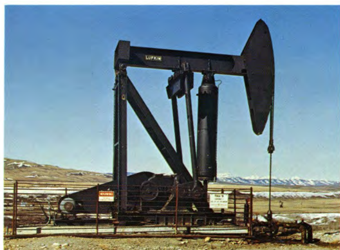
LUFKIN A-456D-144-34.2 Unit, Western Decalta Petroleum Ltd., Turner Valley, Alberta, Canada.
