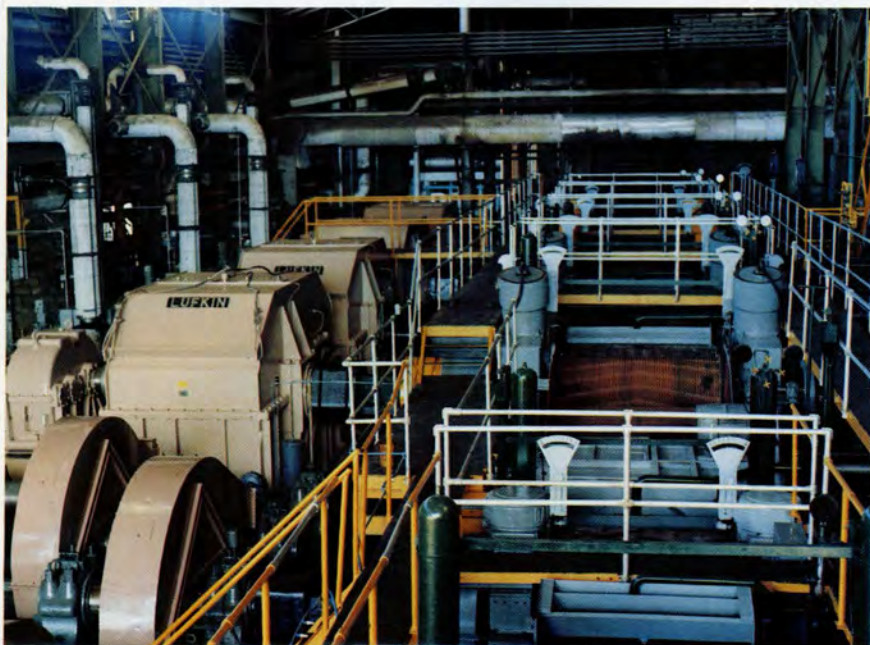
Four LUFKIN N440C Gear Reducers with four LUFKIN DF1070C Double Reduction Gears are driving a FULTON three-roll sugar mill at Ingenio Puga, Mexico.
