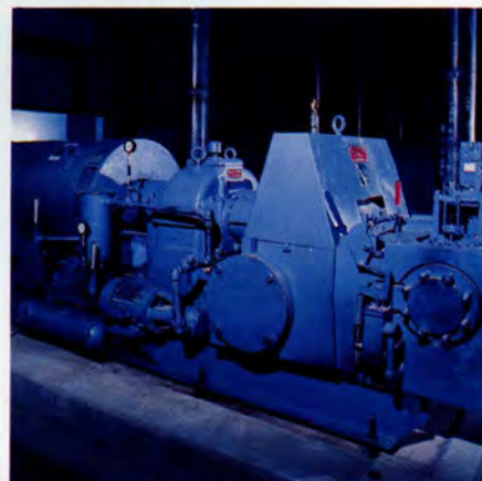
A LUFKIN N1003C Gear Reducer is part of a Trane Murray TMD Turbogenerator installation in a Gin near Bakersfield, California.
