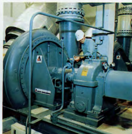
These two single-stage Allis-Chalmers centrifugal compressors are installed in a southeastern sewage plant and used in an aeration process. They are driven by an induction motor rated at 1,300 HP through a LUFKIN N1002C Gear Increaser at 5,650 RPM.
