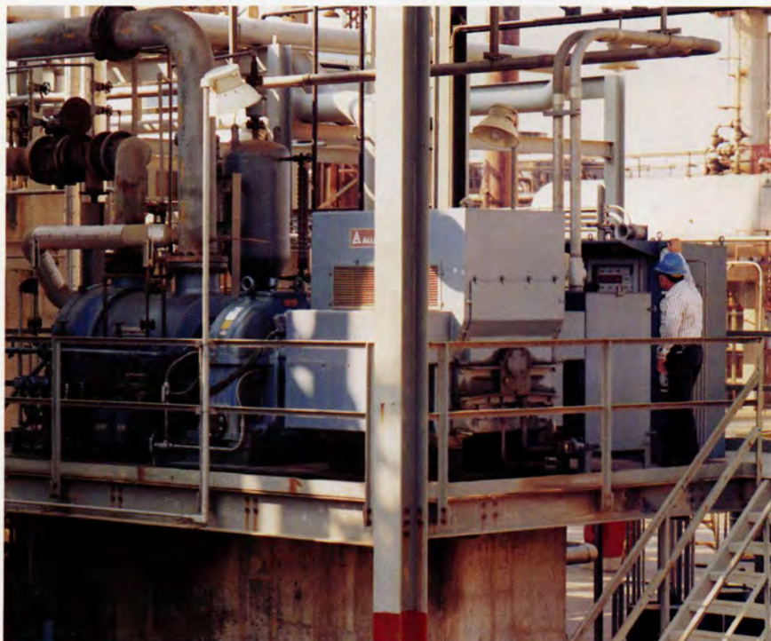
This multistage barrel-type compressor is driven at 10,700 RPM through a LUFKIN N1800C Gear Increaser by a 2,400 HP motor. The unit recycles hydrogen in a petroleum refinery.
