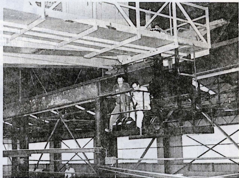
ONE of the cranes is operated by LEAMON BULLOCK, extreme right. Electrician CECIL WALLACE is talking about the operation of the crane which is the very latest design for precise lowering of loads and spotting at designated point. J. E. HOLIDAY, plumber, is in the lower left of the picture.
