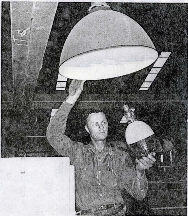
ELECTRICIAN BRYANT CHAMPION is installing the modern mercury vapor lighting which provides maximum comfort and efficiency for workmen.
