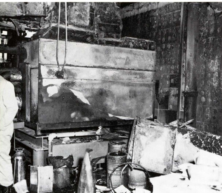
THIS is a partial view of the room which housed the heating and air-conditioning units where it is thought the fire began
