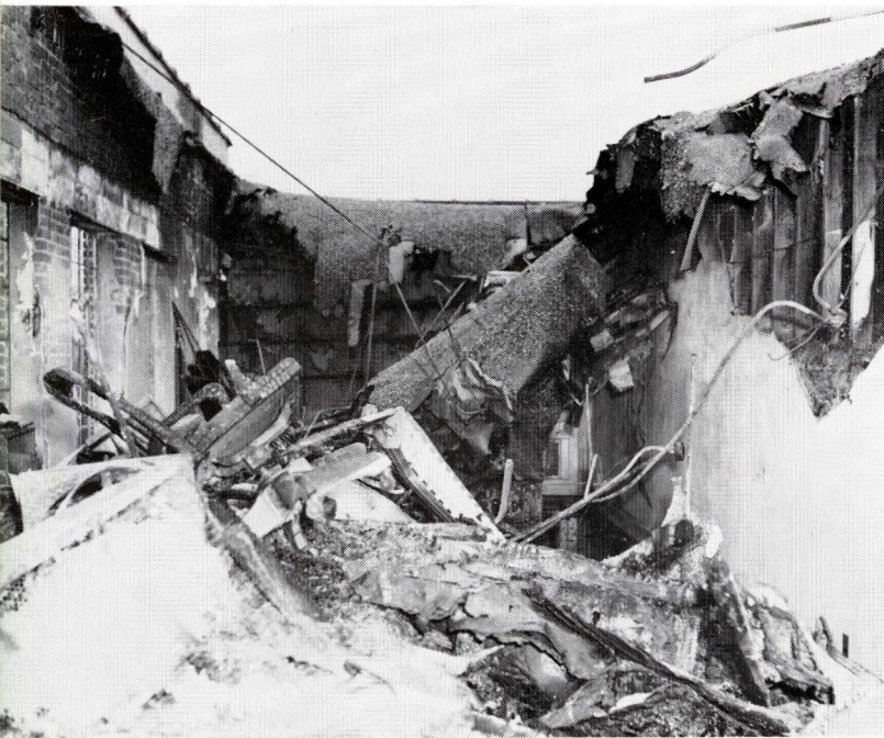
THIS section of the second floor of the Main Office was occupied by the Order department. Some records were lost here but duplicates were in the Material Control department and can be replaced
