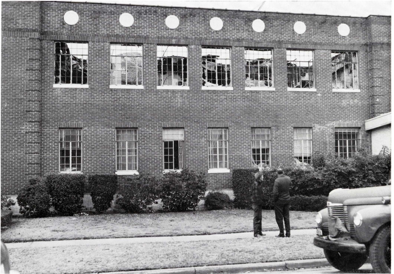
THIS front view of the older section of the Main Office shows the roof caved in on the Order Department located on the second floor.
