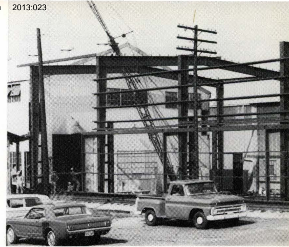
STEEL columns reach toward the sky as the Utility Maintenance crew erect
