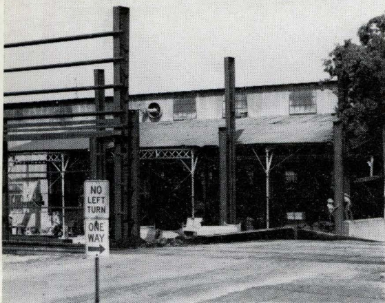
a home for the giant new Schiess gear machine which will arrive in late summer
