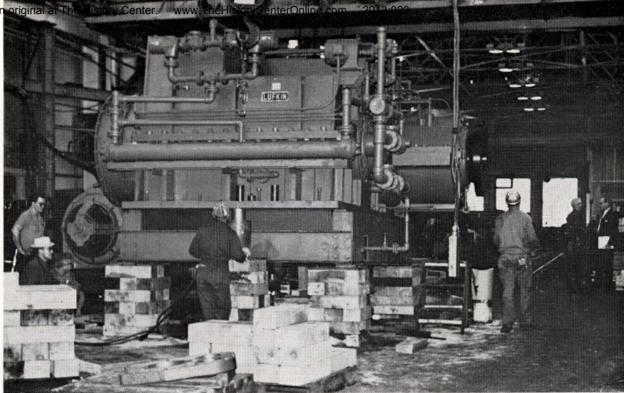
14. THE COMPLETED gear was lifted corner-by-corner and wooden blocks were placed underneath for support. Then the low-boy was backed under the raised unit.
