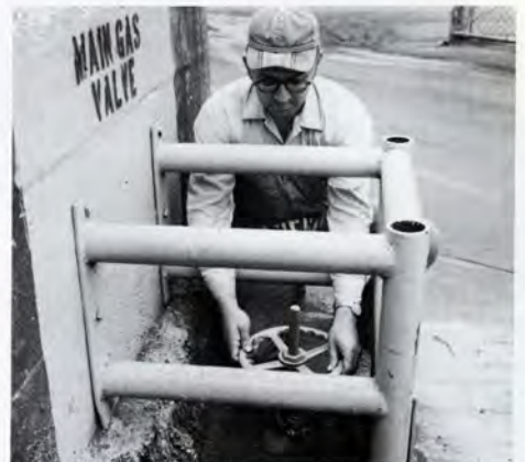
Harold Oldham, utility maintenance, 1st shift, checks to see that the main gas valve located in front of the utility maintenance shop has been cut off
