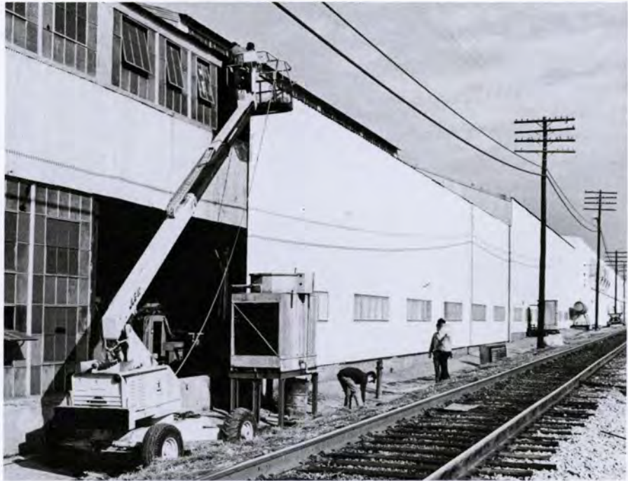
Crews replace windows and tin siding on the machine shop windows adjacent to Angelina Street. The new insulated walls will keep the shop warmer in the winter and cooler in the summer.
