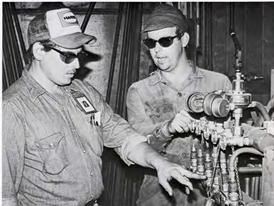
(l-r) David Pleasant and Lawrence Holt check the controls of new gas lines that fuel the torches to preheat gear blanks for welding.
