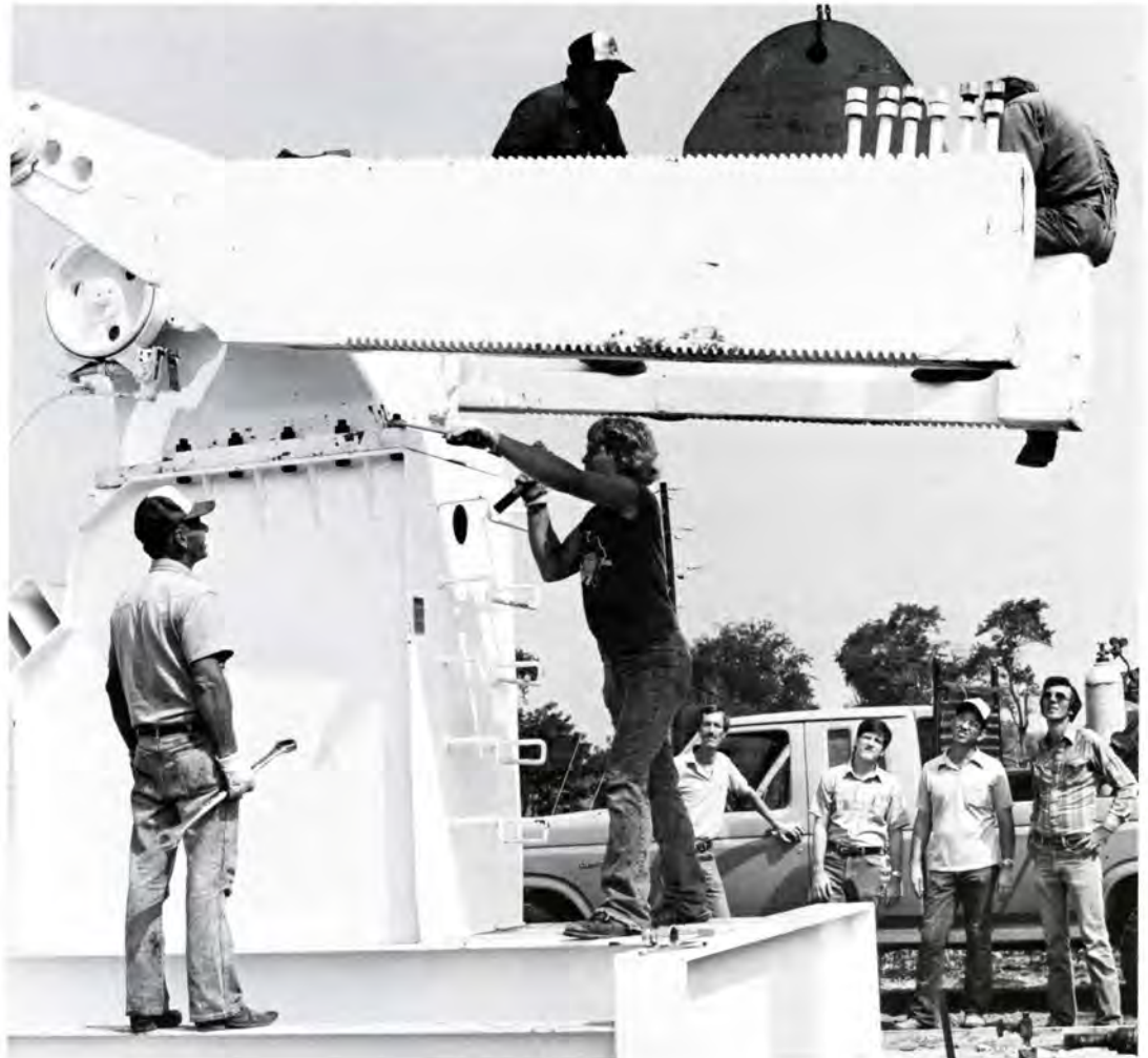
(l-r) Steve Reynolds, Robin Edwards, David Bowers and Robert Nunn watch the installation crew bolt the gear reducer in place.
