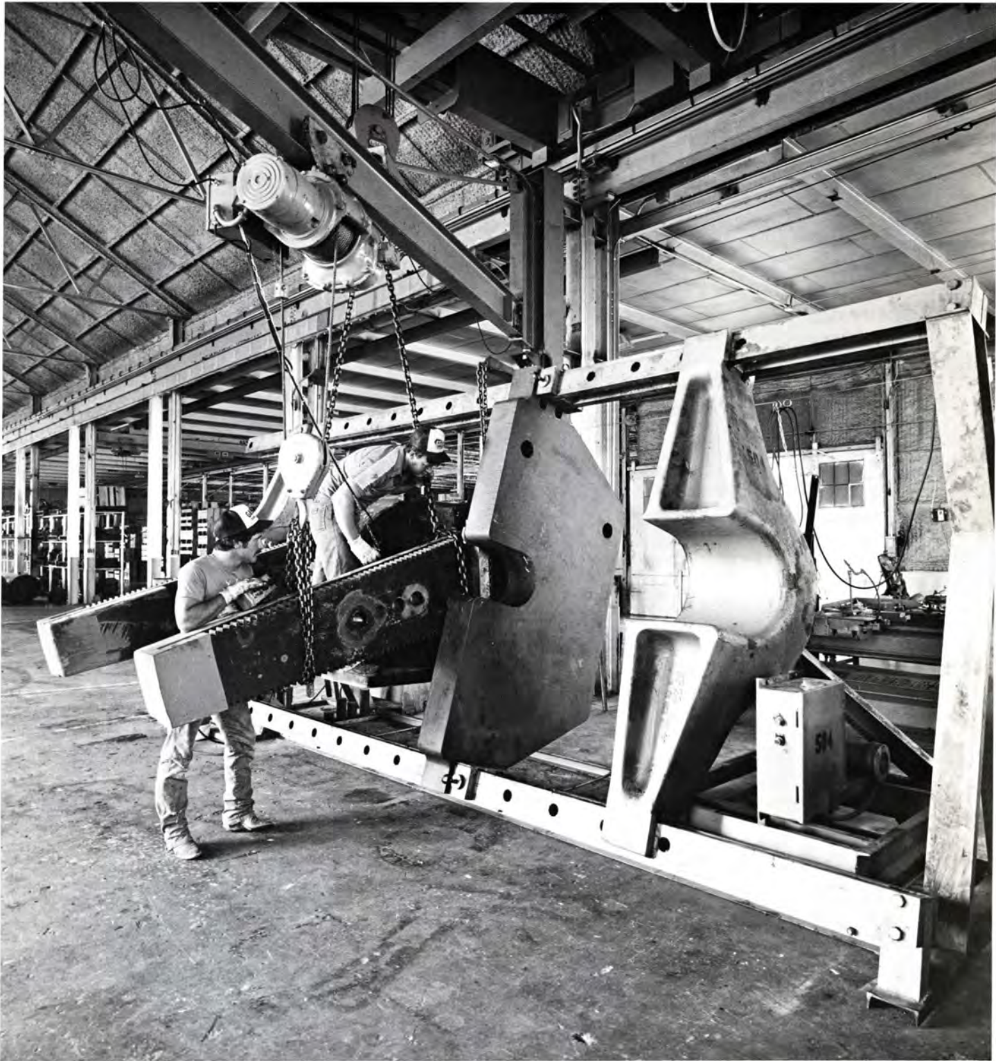
Once turned over to local machine shops, complete overhauls of pumping unit gear boxes are now performed in the Odessa repair shop. Mechanics, Trey Dunson, left, and Lonnie Looney, use the new 400-ton press to remove cranks and replace damaged slow speed gear. (Opposite page, top) Lonnie sets up a job on the new key-shaper. (Bottom) Lonnie, left, and Trey replace the high speed bearings on a LUFKIN gear box.
