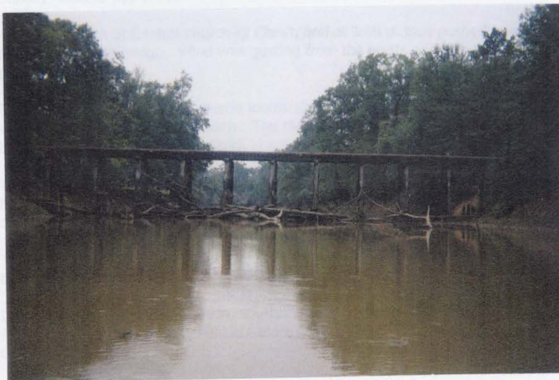
Log jam at abandoned TSE trestle
